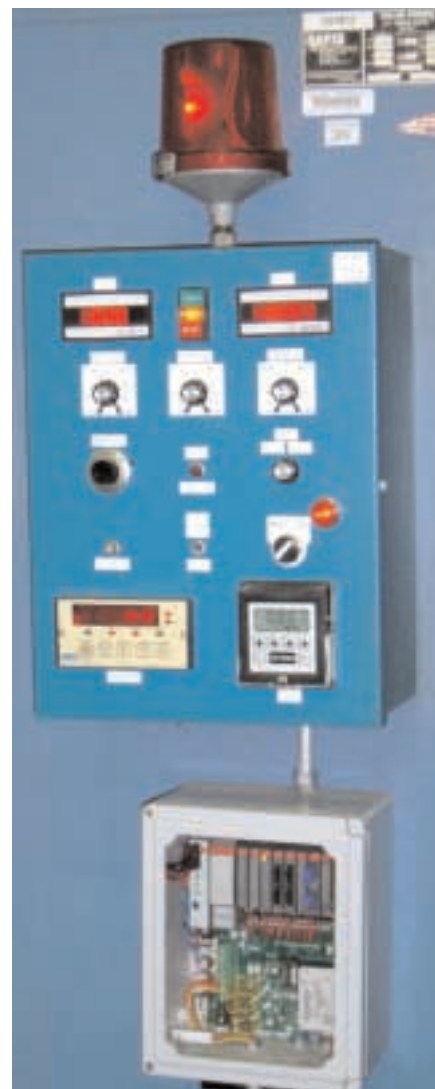
Metalast™ Interface Controller shown underneath existing Rectifier Control Panel which monitors and controls system power outputs.
